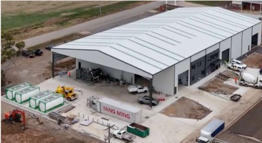
Maddingley -Advanced Recycling Plant
